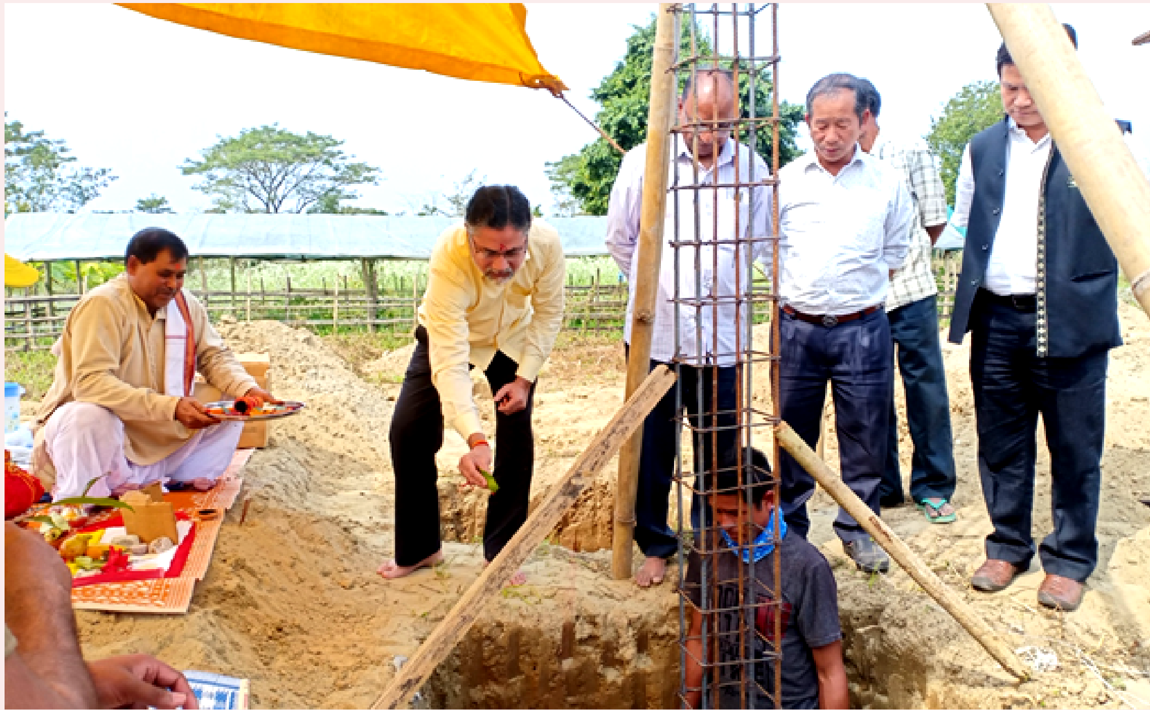
Dr. Dhanjay Kulkarni laying the foundation stone for the Arogya Center on Feb 21 2020 in Arunachala Pradesh, India.
