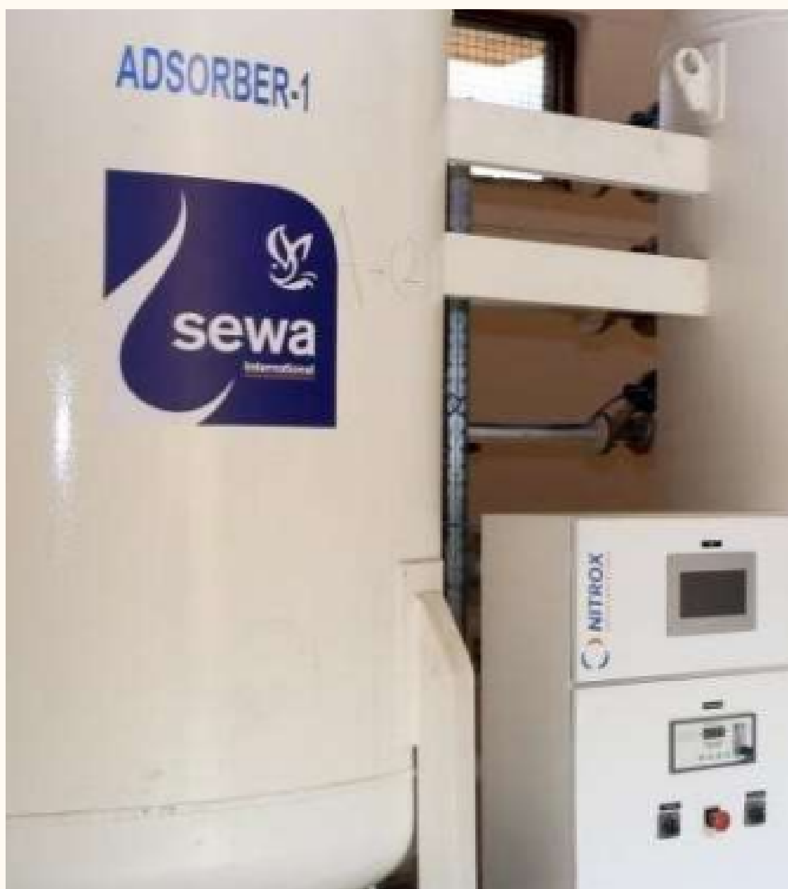
A picture of an Oxygen (O2) Generation Plant installed in a rural hospital by Sewa International in India
